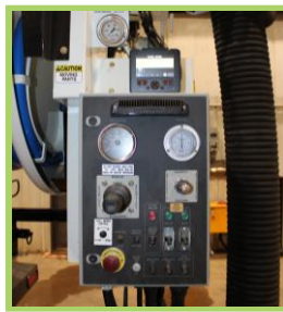
Rear Operator Controls
