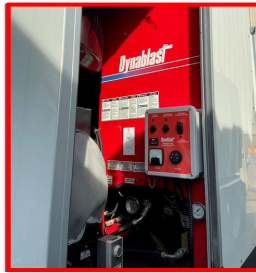
700K BTU Hot Water Heater
